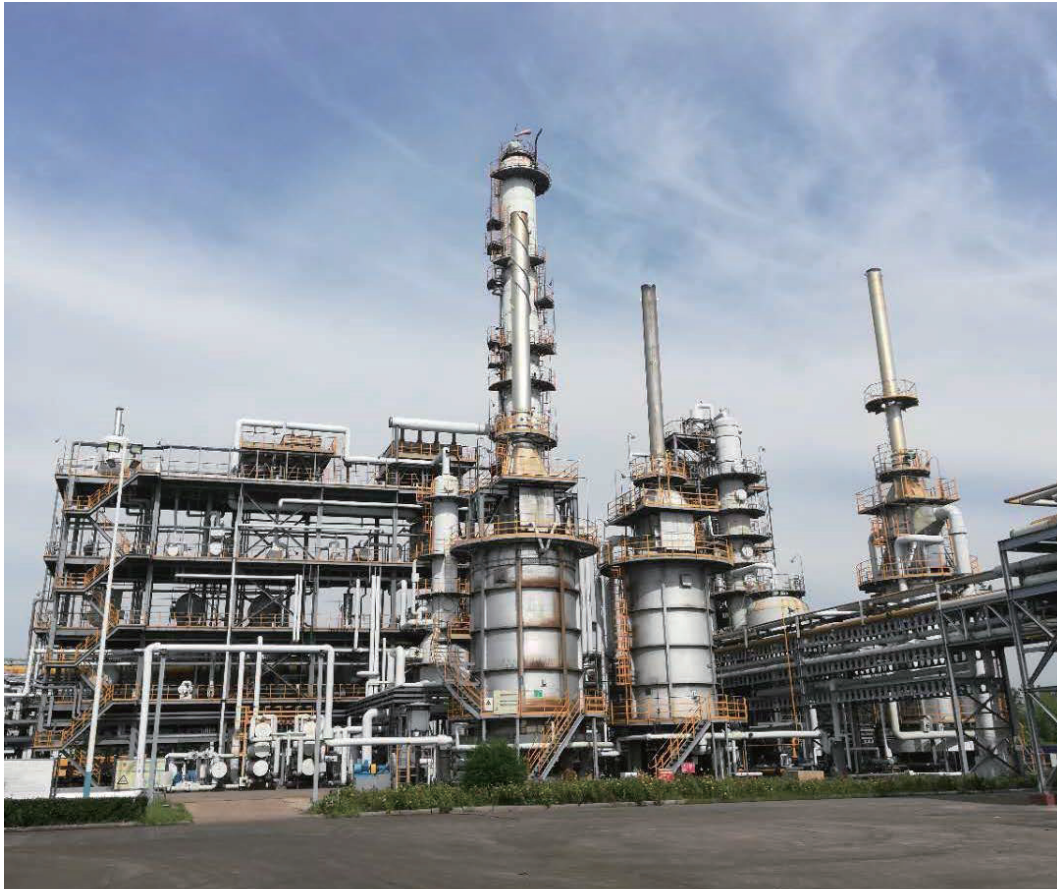
Coal tar processing facilities at our Xingtai Production Base
